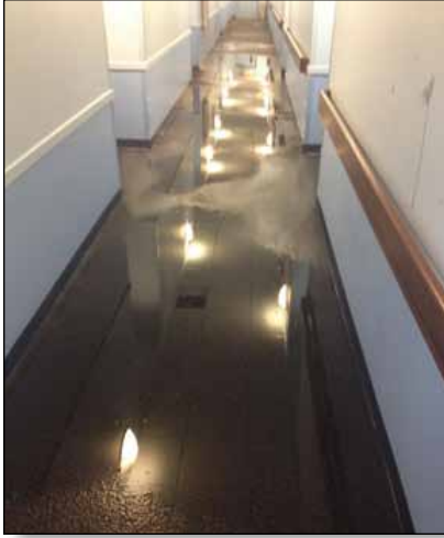
The flooded hallways at Covenant Harbor in Oak Harbor made it necessary to temporarily move residents.
